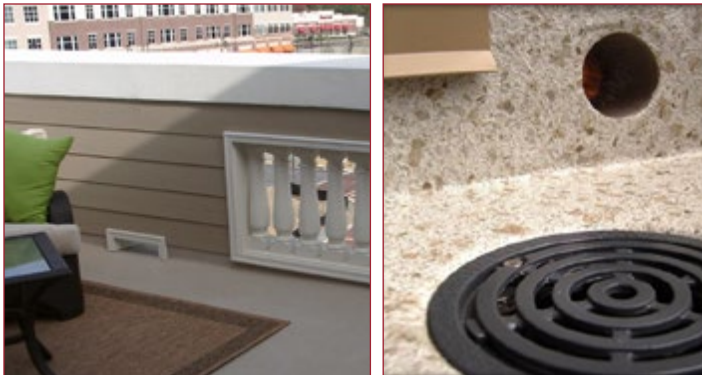
Slope, drains and PVC Coated Scuppers allow water to drain off a trapped deck.
