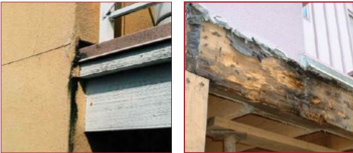
Severe structural damage can occur when water is not properly diverted.
