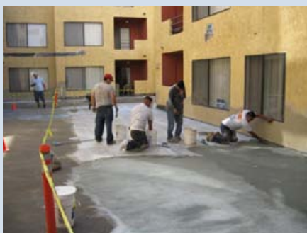
Photo courtesy Central Coast Waterproofing
