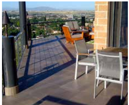
The flexibility of TileDek allowed the installer to wrap the columns and prepare them for tile installation.
