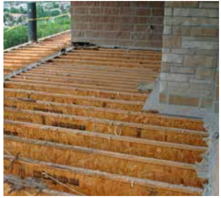
Ineffective waterproofing on upper and lower level decks in this Odgen, Utah home caused extensive water damage and the need to replace the substrate.
