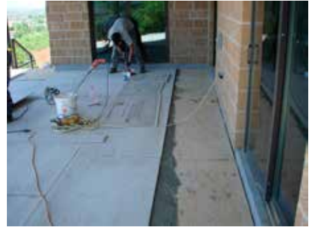
After replacing the substrate, MBL Construction readied the surface for tile by installing the TileDek membrane, tile backer and bond coat of MAPEI Ultra Flex 2 .
