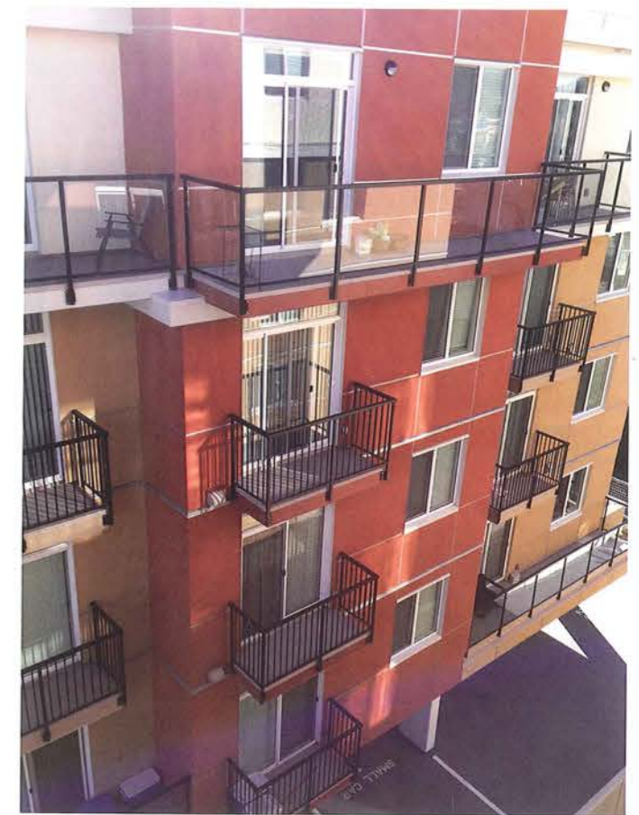
These balconies are covered in a vinyl membrane: attractive, low maintenance, and safe.
