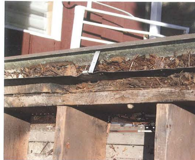
The wood rotted from water infiltration caused by inadequate waterproofing.
