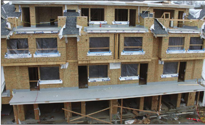
This image illustrates sequencing to integrate polyvinyl chloride (PVC) roof membrane with the building envelope.
